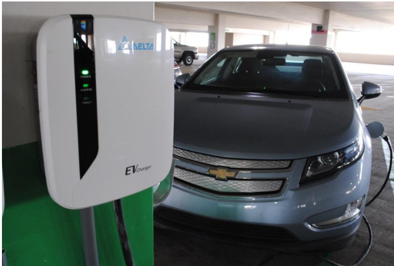
Photo of the 2nd generation EVSE Prototype installed and under field trial at DTE's parking garage in downtown Detroit, MI.
