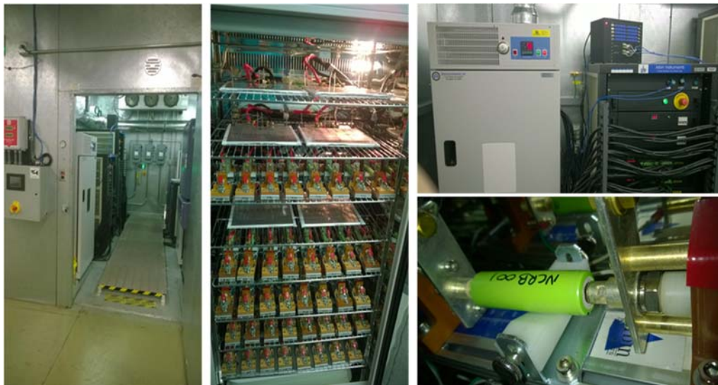
Figure 1 - Battery testing laboratory entrance, inside temperature chamber, temperature chamber and battery tester & a commercial “18650” Li-ion cell used for the EVTC project in battery holder. (Photos: Dr. Arnaud Devie, HNEI)
